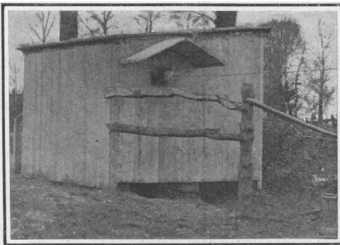
Transformer Shed and the Wire Which Carries 100,000 Volts, Direct Current, to the Field and Stimulates Plant Growth.
