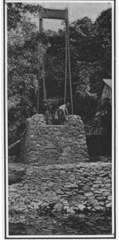
The Towers Consist of Four 70-Pound Railroad Rails Set in a Concrete Base.
