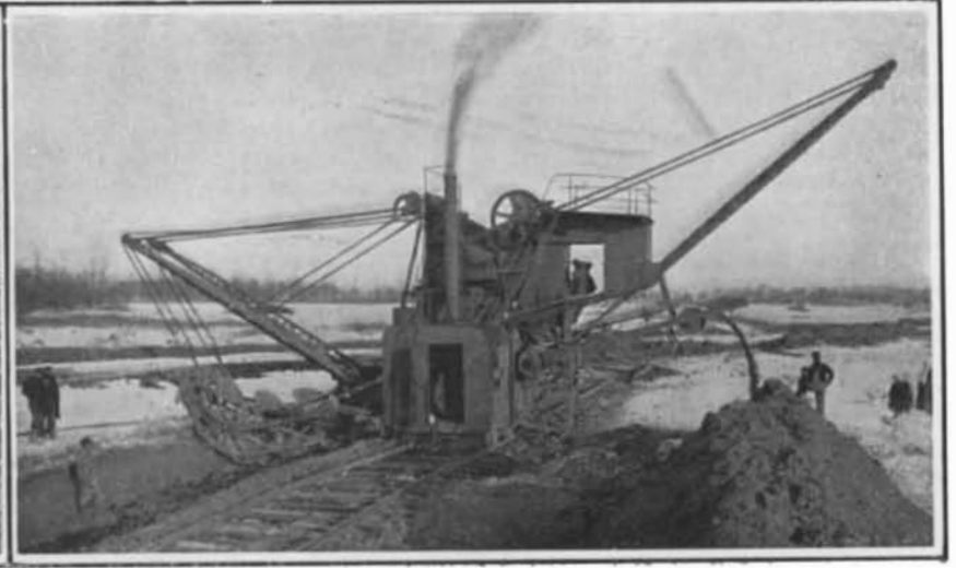
Lubecker Excavator. The Material is Dug from the Left-Hand Side of Machine, Emptied onto a Conveyor, and Deposited in Dump at Right.
