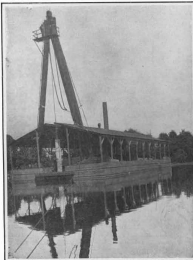
Loentz Rock Breaker. Operated by Lifting and Letting Fall the 16-Ton Iron Hammer Seen Below the Derrick.
