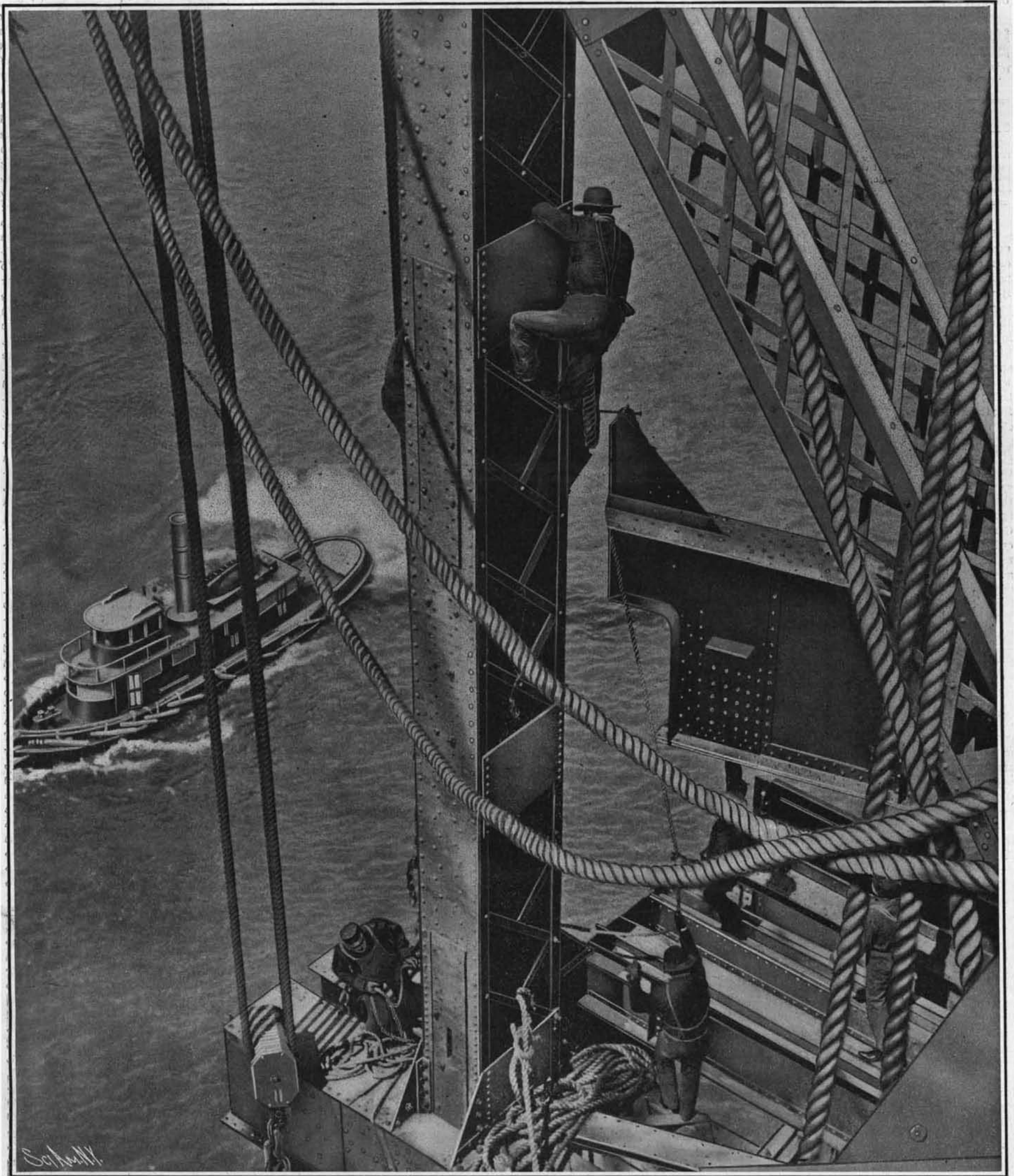
At Work Erecting the Cantilever. The View is Taken 160 Feet in Mid-Air and 500 Feet Out from the Point of Support.
