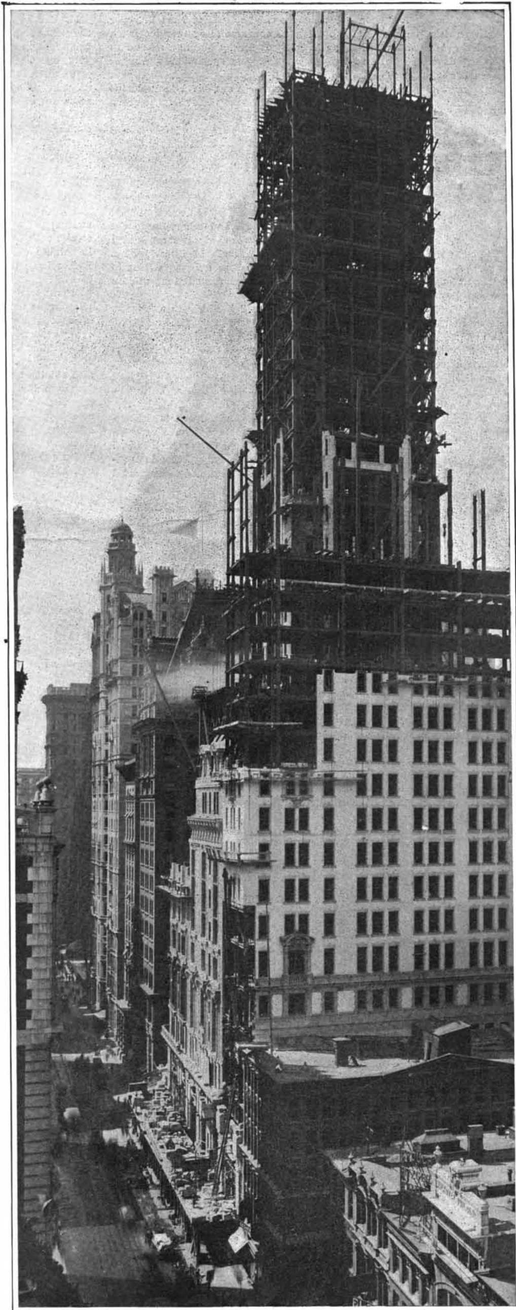
The Top of the Projecting Columns is 500 Feet Above Street Level. Note the Wind Bracing in the Side Panels.
