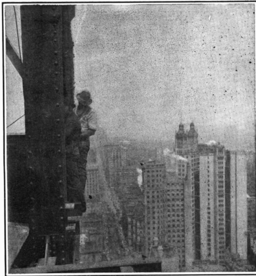
Working on a Corner Post of the Tower at the 450-Foot Level.
