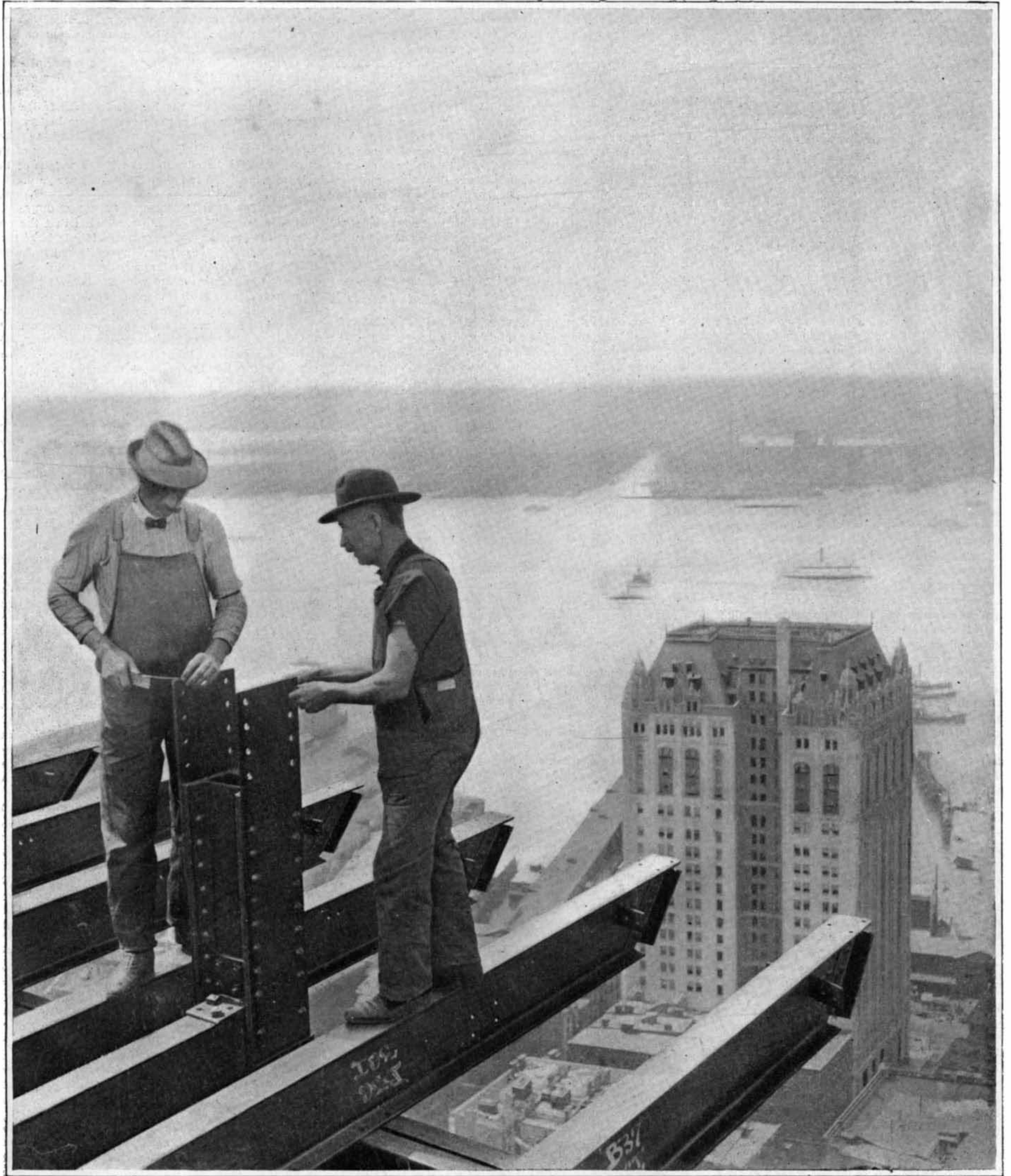
Preparing to Erect a Steel Column at the 500-Foot Level of the 612-Foot Singer Building, New York.
