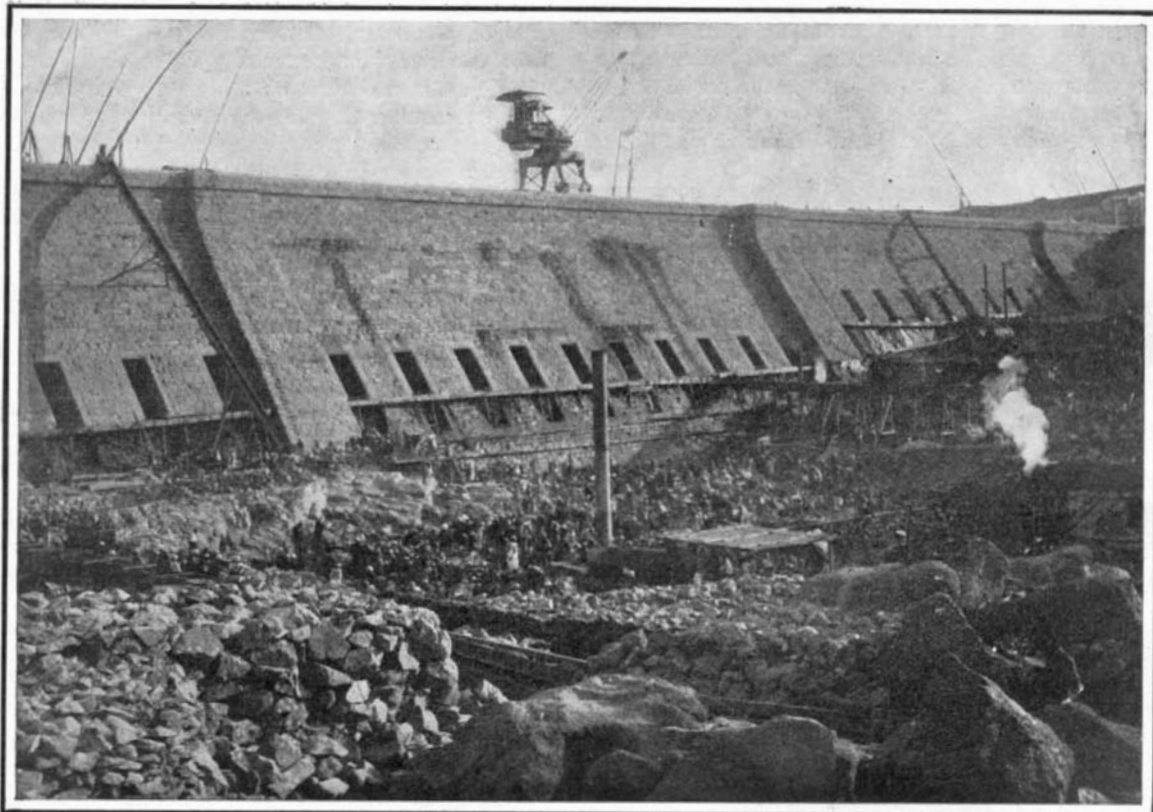
Excavating 350,000 Cubic Yards of Loose Rock and Gravel from the River Bed, Preparatory to Building the Masonry Apron.
