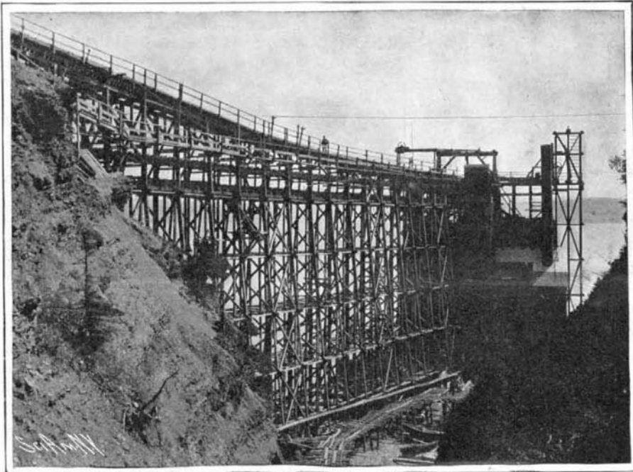
Iron Ore Shipping Pier at Belle Isle. The Ore is Shipped to England and the United States to Be Smelted.
