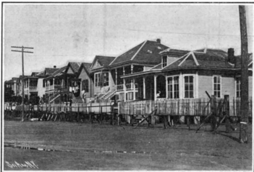
In Raising the City All the Houses Are Elevated on Stilts and the Dredgers Fill under Them. The White Mark on the Telegraph Pole Shows the Final Grade.
