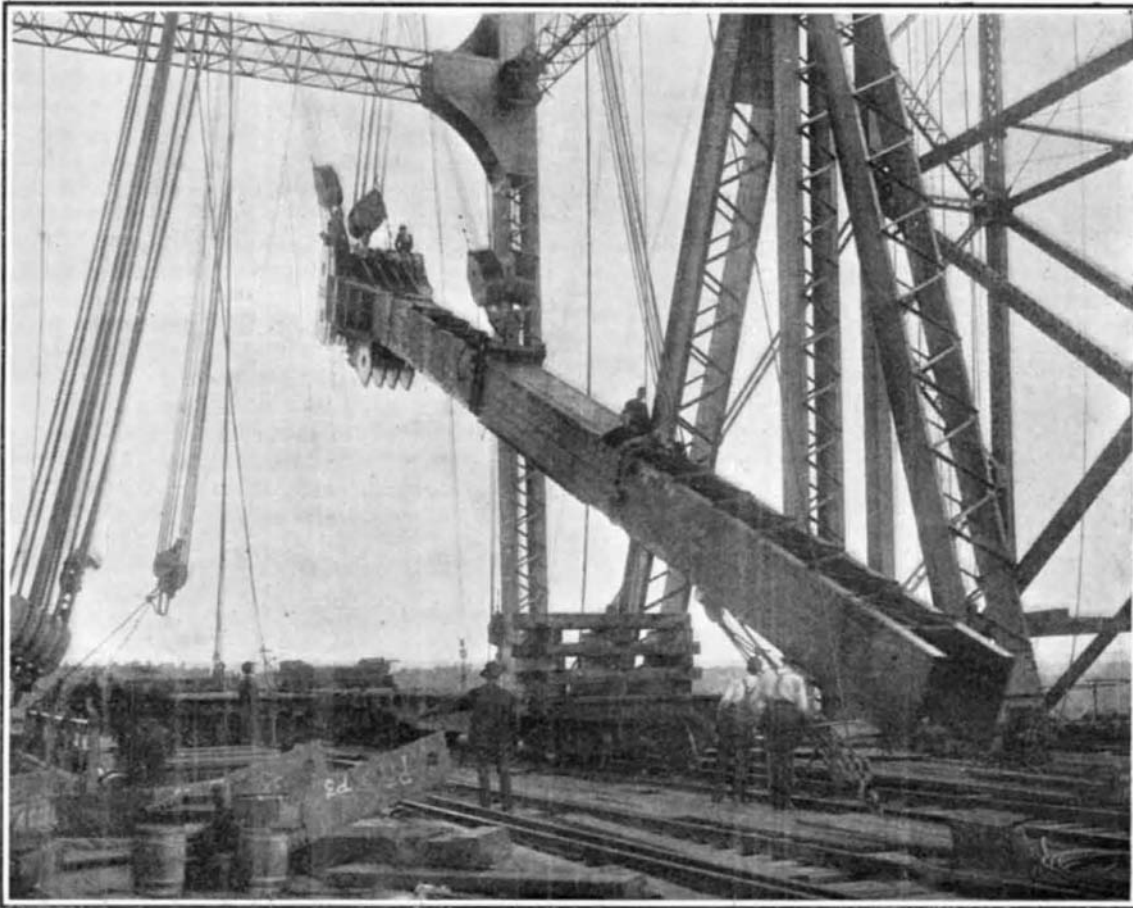
Raising the Top Section of the First Main Intermediate Post of the Cantilever Arm, Quebec Bridge.
