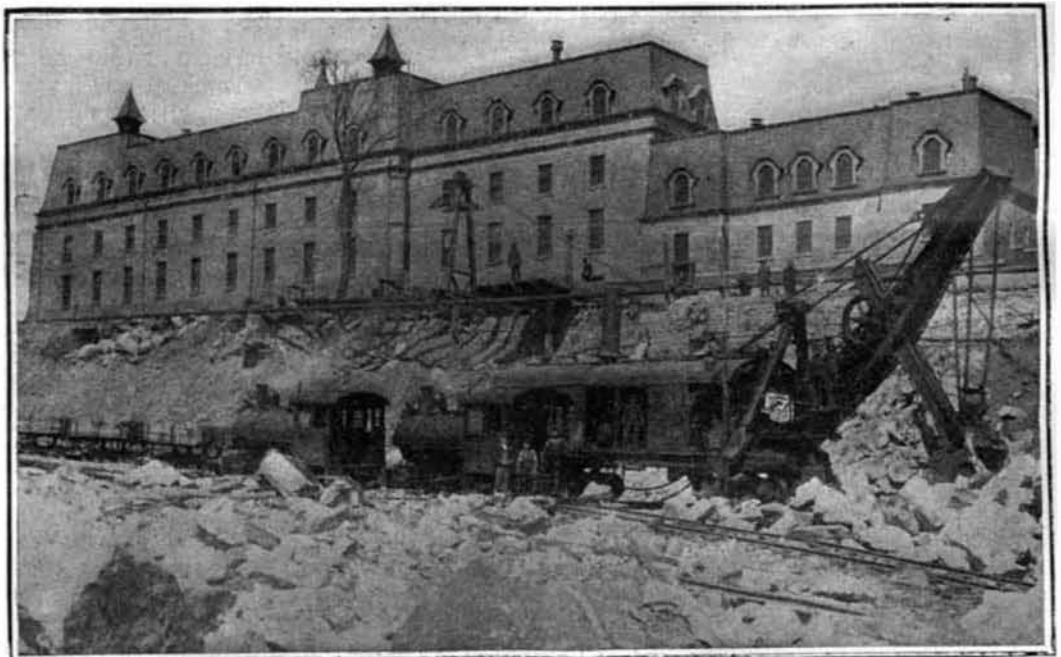
Seventy-Ton Steam Shovel Working on Northerly Side of Excavation at 33d Street.
