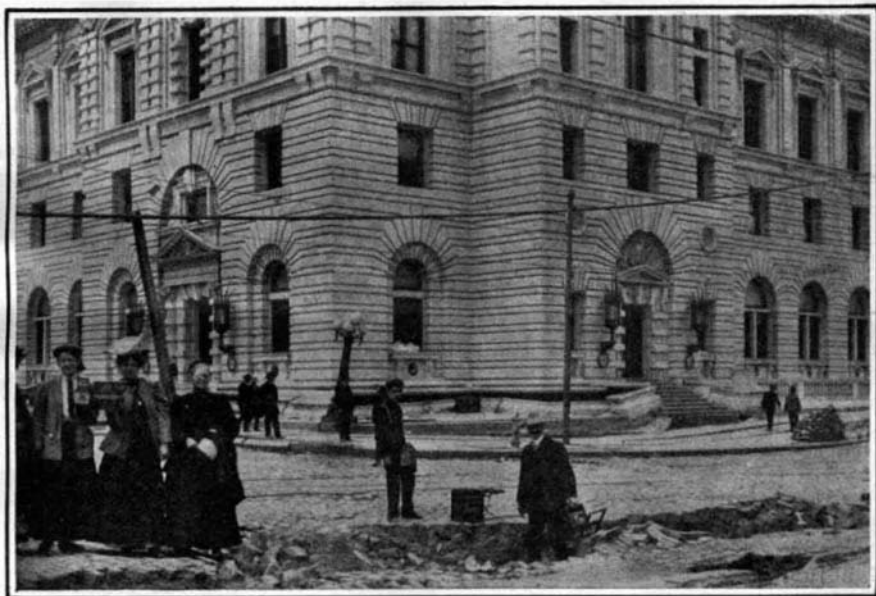
The Post Office Suffered Little. Only Sidewalks Are Twisted. Note Fissure in Which Man Stands.
