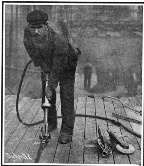
PNEUMATIC DECK-CALKING TOOL IN OPERATION, SHOWING SEAM OPENER AND CALKING IRON WITH PNEUMATIC HAMMER.
