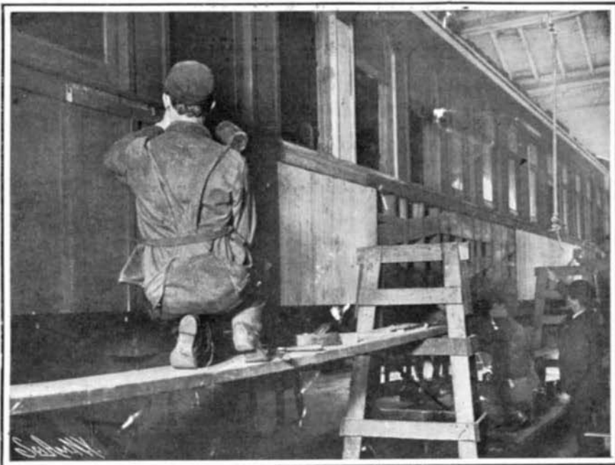
Putting the Siding on a Skeleton Car Body and Hanging the Piping.
