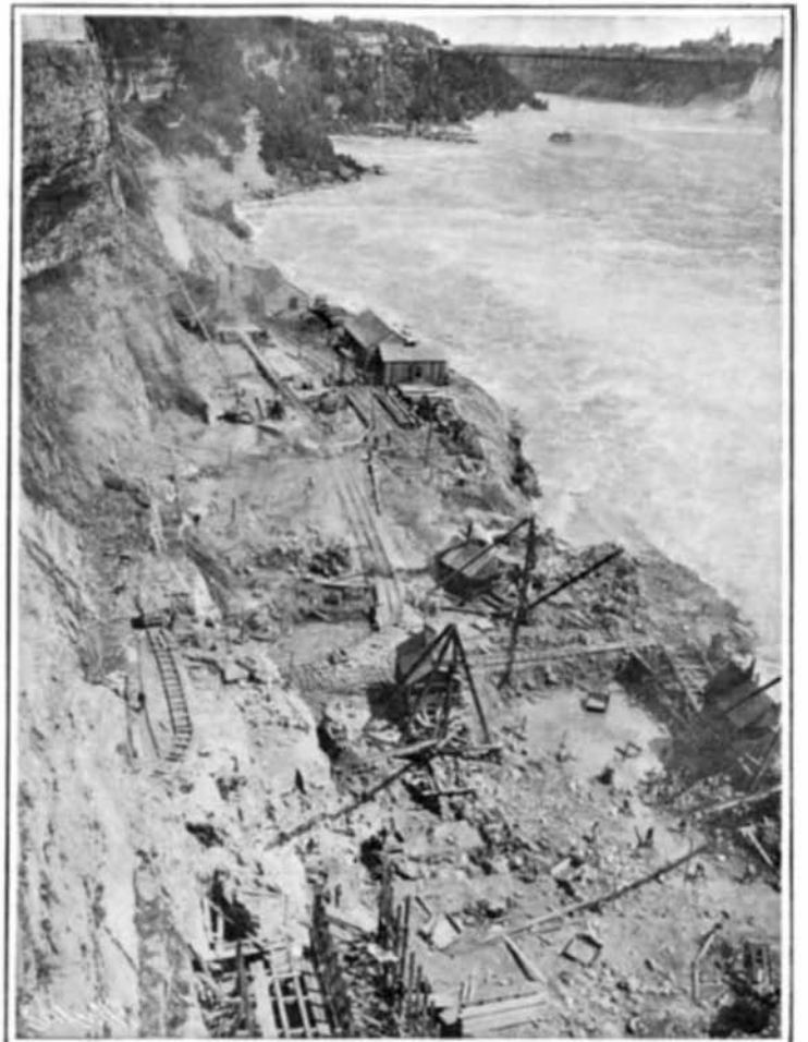
Excavating the Site for the Generating Station at the Foot of the Cliffs.
