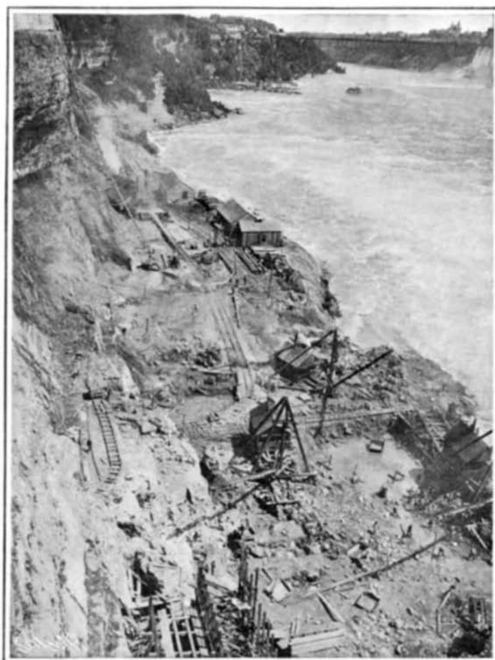
Excavating the Site for the Generating Station at the Foot of the Cliffs.
