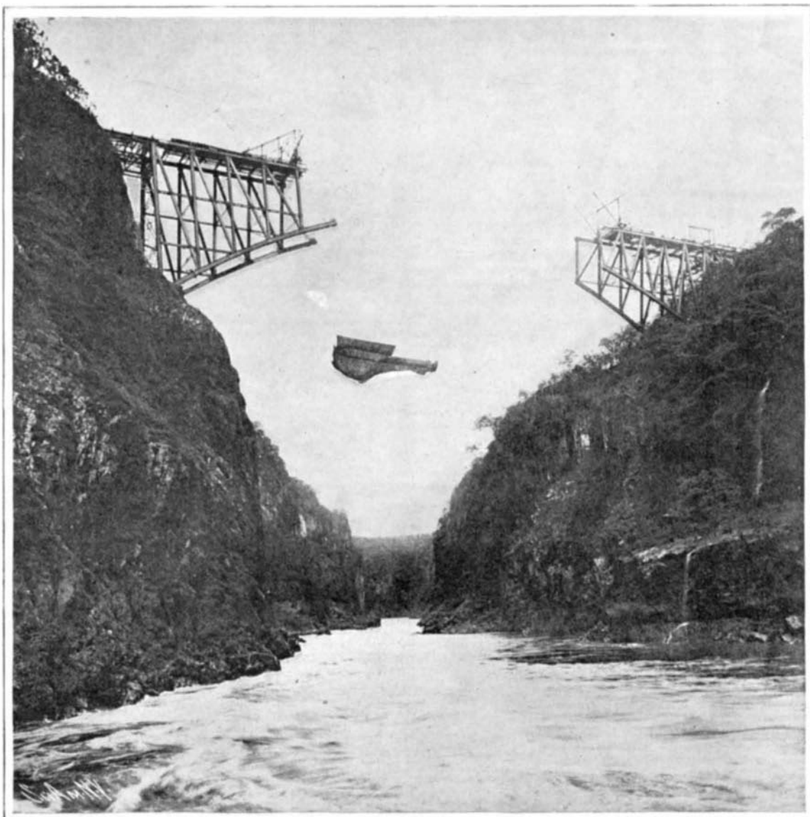
THE VICTORIA FALLS BRIDGE IN COURSE OF ERECTION. THE MATERIAL WAS CARRIED BY CABLEWAY.
