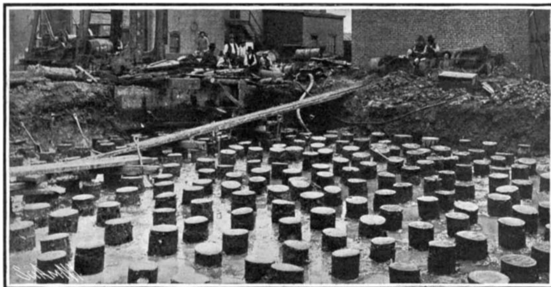
Excavation 4 Feet Below Grade, with Piles Cut Off 3 Feet Below Grade, Ready for Concrete.
