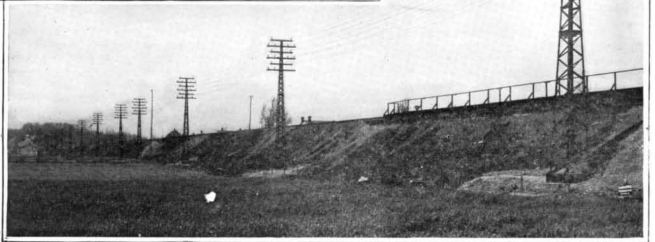
View of Trunk Transmission Line Between Long Island City and Woodhaven Junction, Showing Latticed Steel Poles.
