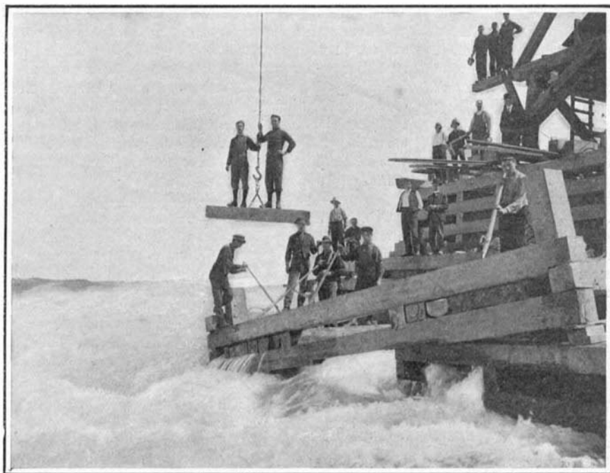
Launching a crib in 26 feet of water in the upper rapids where the water is running at 15 miles an hour.
