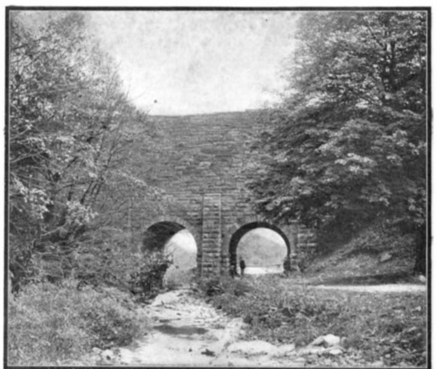
MASSIVE STONE CULVERT, RECENTLY DESTROYED. ERECTED IN 1848 ON THE LINE OF THE NEW PORTAGE RAILROAD.
