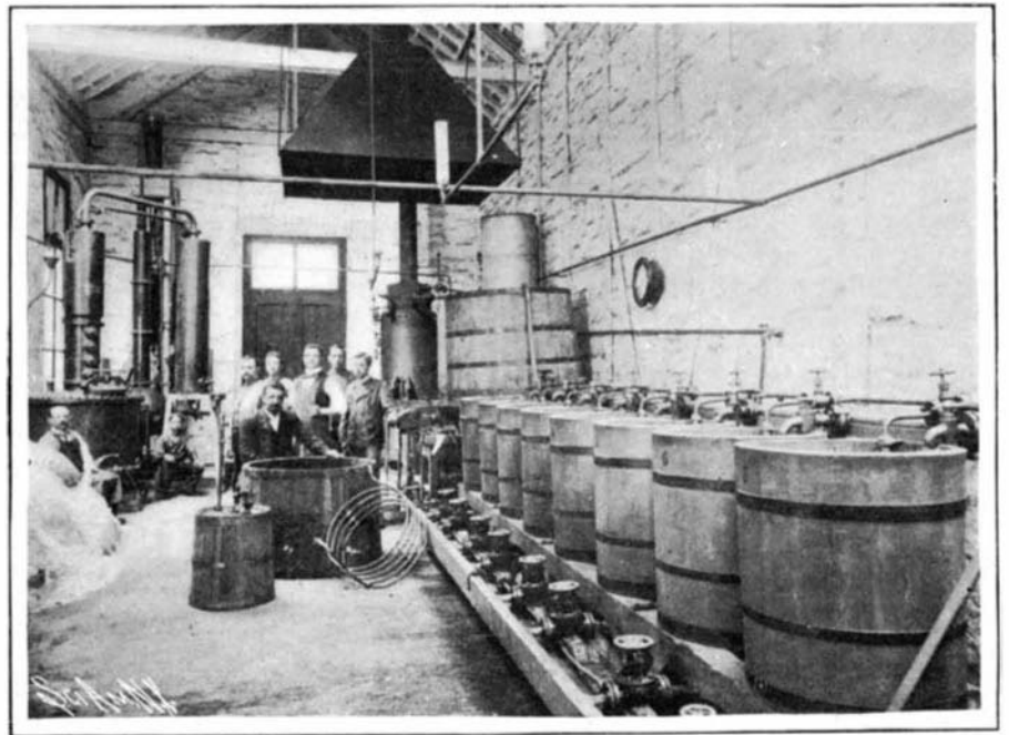
At the right: Exhauster for extracting sugar formed in digester. At the left: Alcohol stills.
