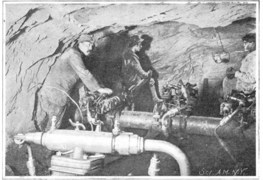
Three Brandt Hydraulic Rock Drills, with Which all the Rock-Drilling Was Done.
