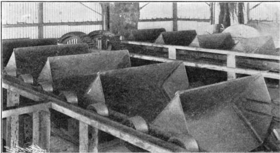
Overhead Horizontal Runs of Gravity Discharge Elevators from which Coal is Spouted to Belt Conveyor.
