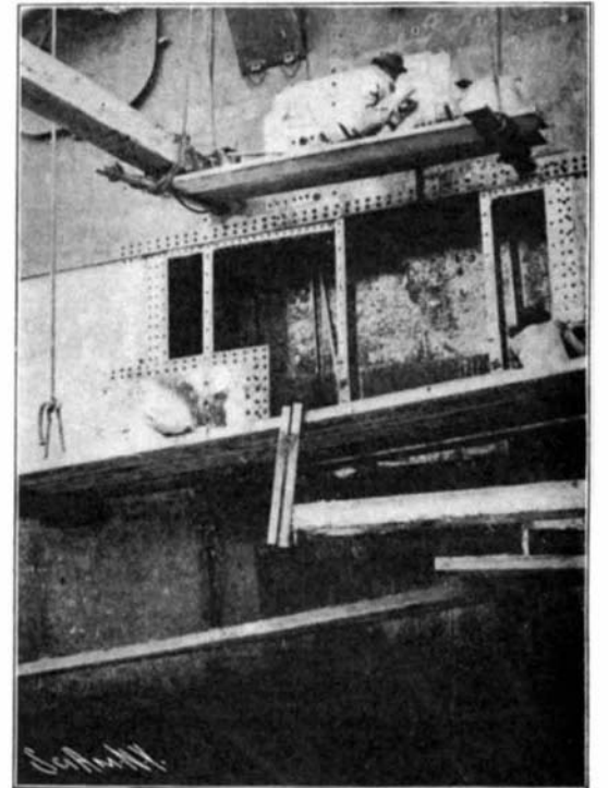
Damaged Plating Removed Preparatory to Replating.
