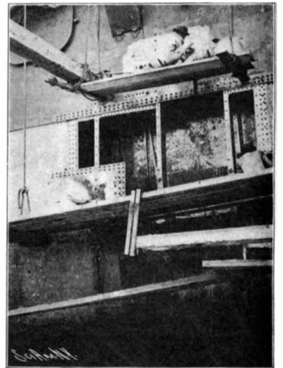
Damaged Plating Removed Preparatory to Replating.
