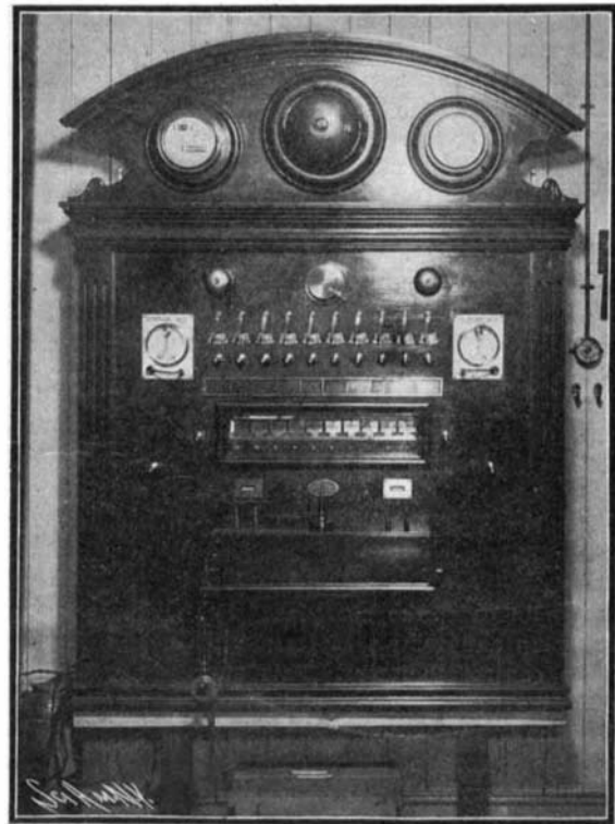
Fig. 2.—Fire Alarm Switchboard.
