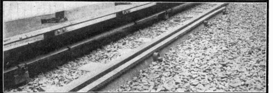
Section of Third Rail with Covering Board in Place
