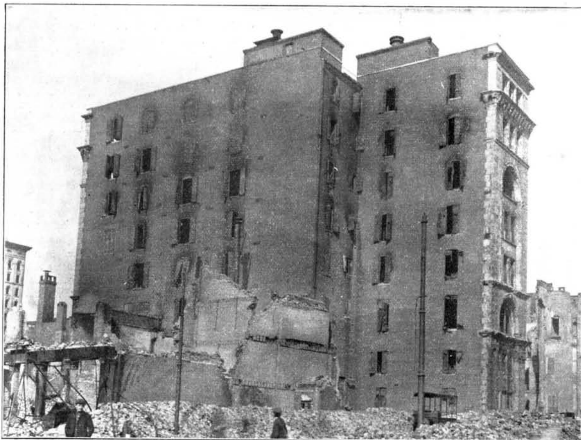
Merchants' National Bank, Showing Sheet-Iron Shutters Burst Open by the Sudden Combustion of Gases Within the Building.
