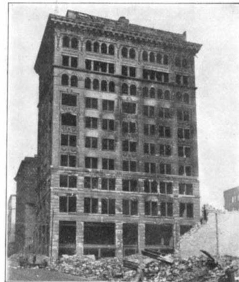
Union Trust Building, Showing the Severe Spalling of the Stone Facing.
