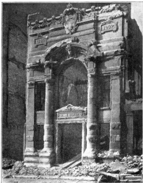
New Banking House, Showing Action of Fire on Sandstone Front.
