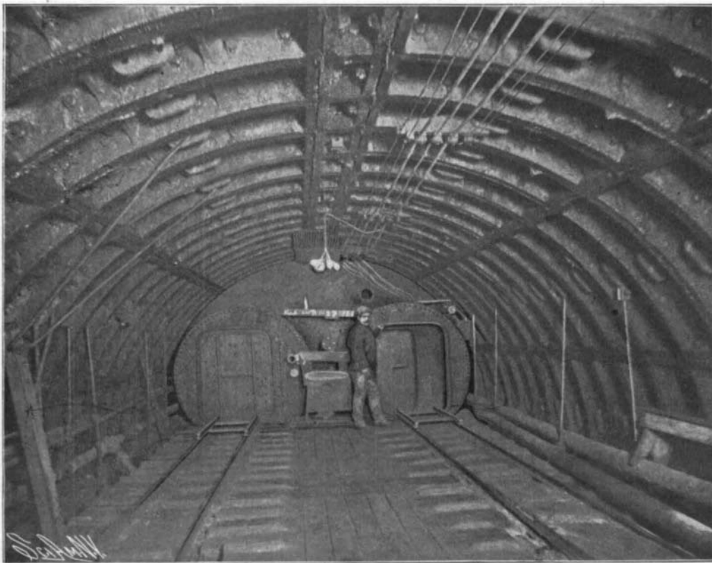
View of Twin Air-lock in Tunnel, Showing Shifting Rails for Entering Lock Chamber.
