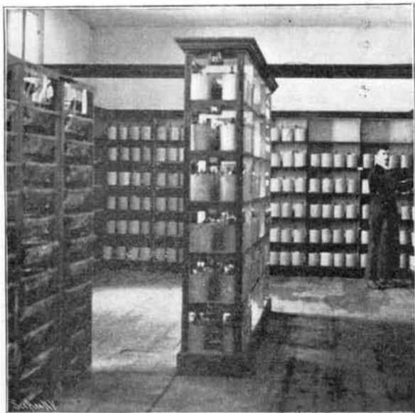
A Corner of the Battery-Room at Heart's Content.
