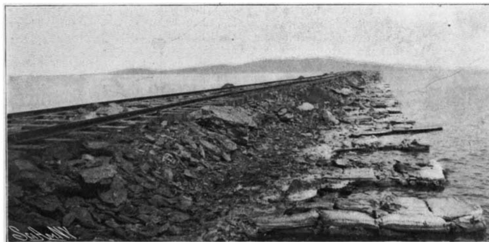
Construction in Shallow Water, Showing Sandbags and Planking Used to Sustain the Temporary Track. Sections of the Permanent Track Have Been Depressed by the Settling of the Roadbed.
