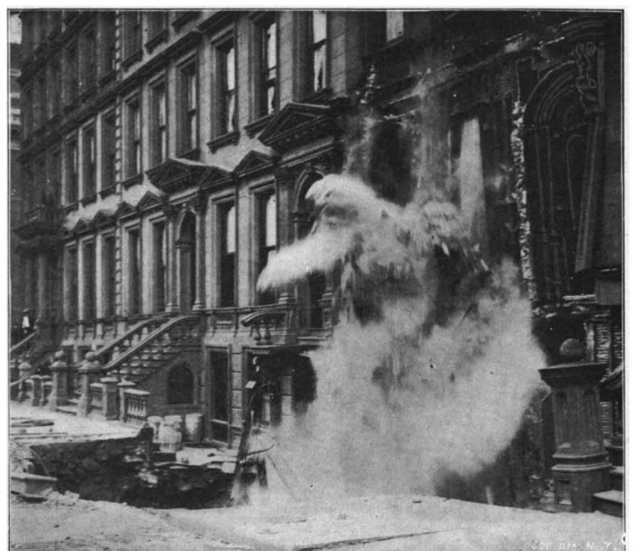
Snapshot Taken as the Front Walls Collapsed.
