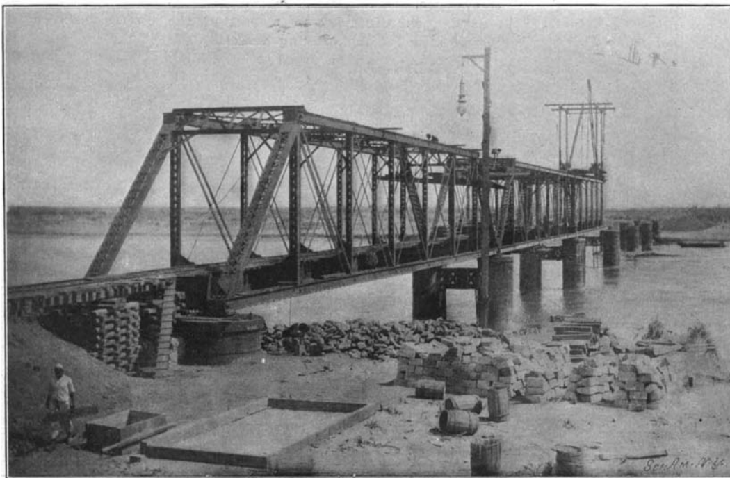
Seven 147-foot spans; total weight of superstructure, 620 tons. Order received January 20; structure shipped March 7; erection completed August 19.
