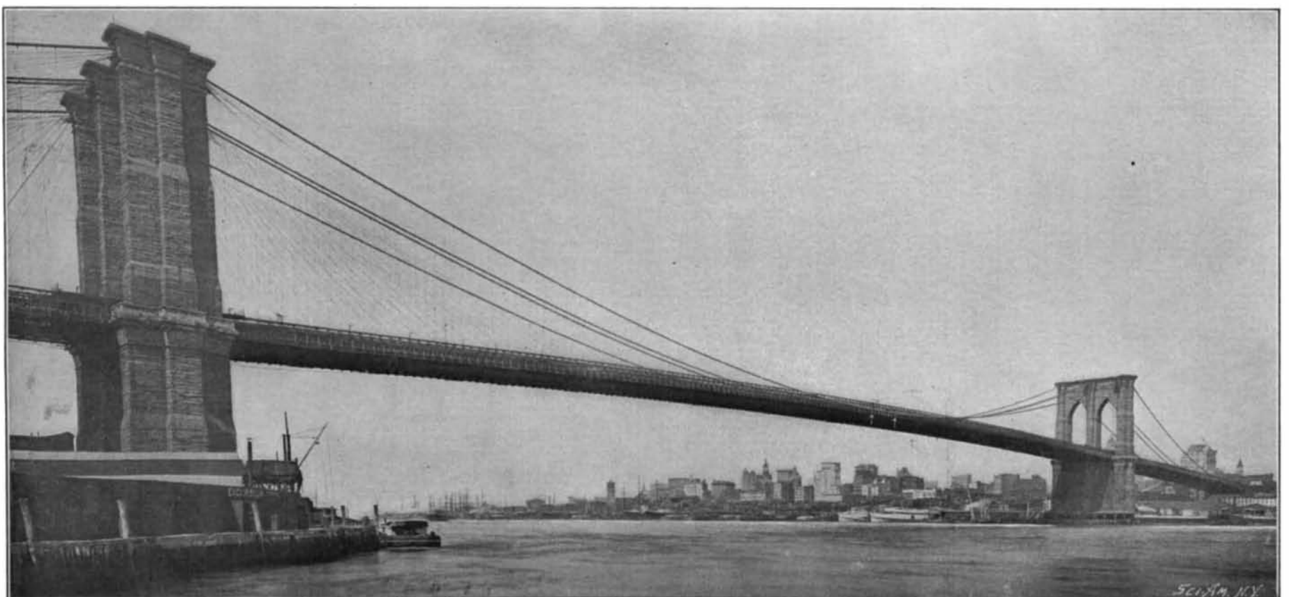
BROOKLYN BRIDGE FROM THE NORTH, SHOWING BY ARROWS AT CENTER, LOCATION OF THE NINE BROKEN SUSPENDERS.
