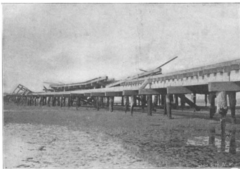
WHARF DESTROYED BY TEREDOS.
