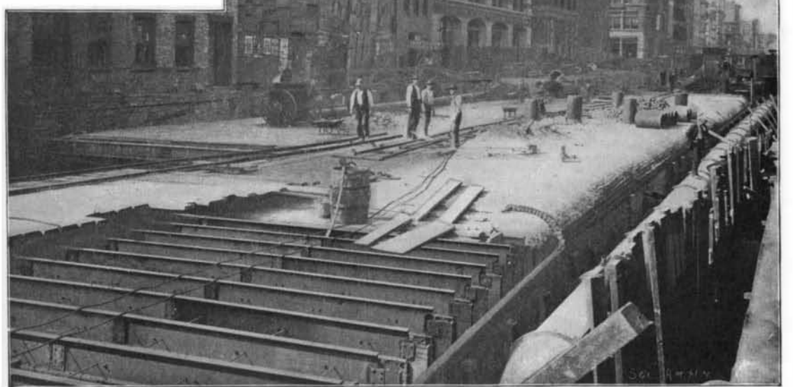
View at Houston and Elm Streets, Showing Brick and Concrete Covering Being Laid Over Steel Work.
