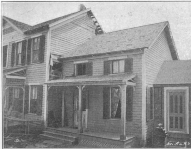
EFFECTS OF LIGHTNING, SHOWING WHERE THE BOLT ENTERED AT THE ROOF AND WHERE IT LEFT THE HOUSE AT THE SIDE.
