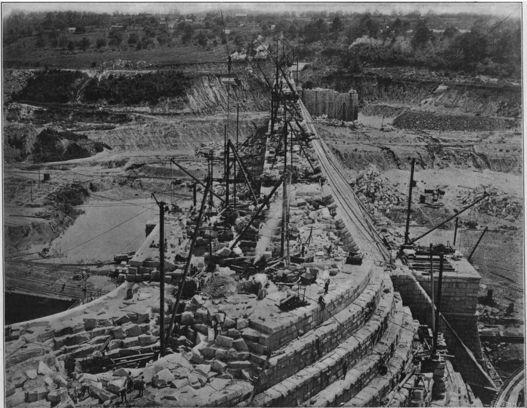
Depth of Foundation Below River, 134 Feet; Width of Dam at Foundation, 216 feet; Height, Foundation to Coping, 300 Feet; Length of Dam on Crest, 1,050 Feet; Length of Spillway, 1,000 Feet.
