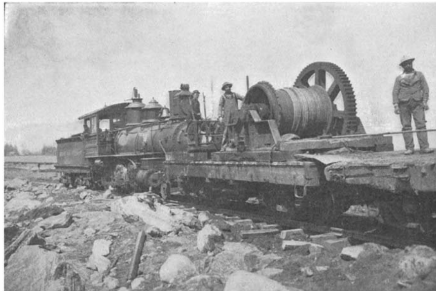
Locomotive and Lidgerwood Hoisting Engine for Pulling Plow Over Train of Flat Cars.
