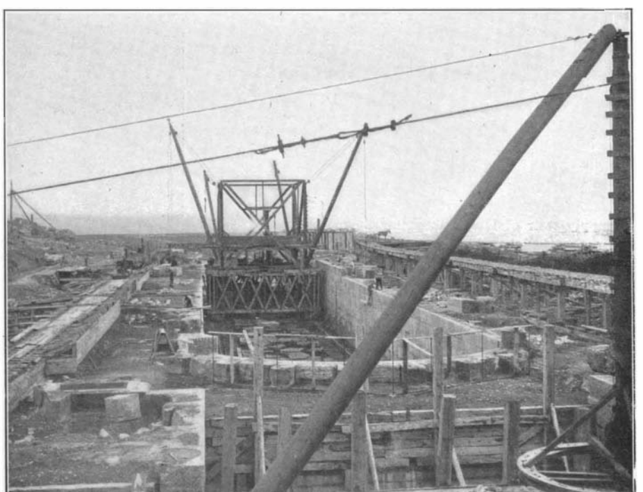
LOCK UNDER CONSTRUCTION—MASONRY PLACED IN POSITION BY DERRICK TRAVELING ON FLOOR OF DOCK.
