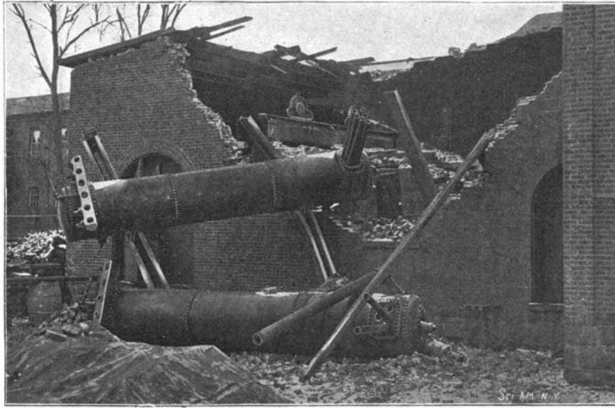
TWO STEAM DRUMS OF A BOILER BLOWN THROUGH BOILER HOUSE.
