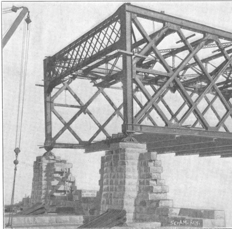
INSHORE END OF THE STIFFENING TRUSSES OF THE NEW EAST RIVER BRIDGE.
