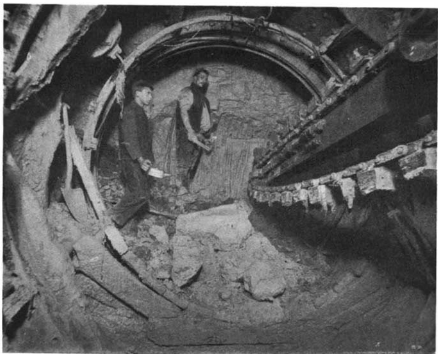
Electric Excavator, Showing the Buckets Working on the Face of the Clay Within the Shield.
