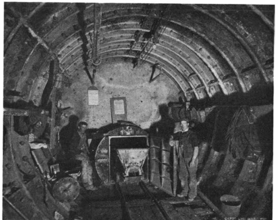
Interior of the Compressed Air Chamber.
