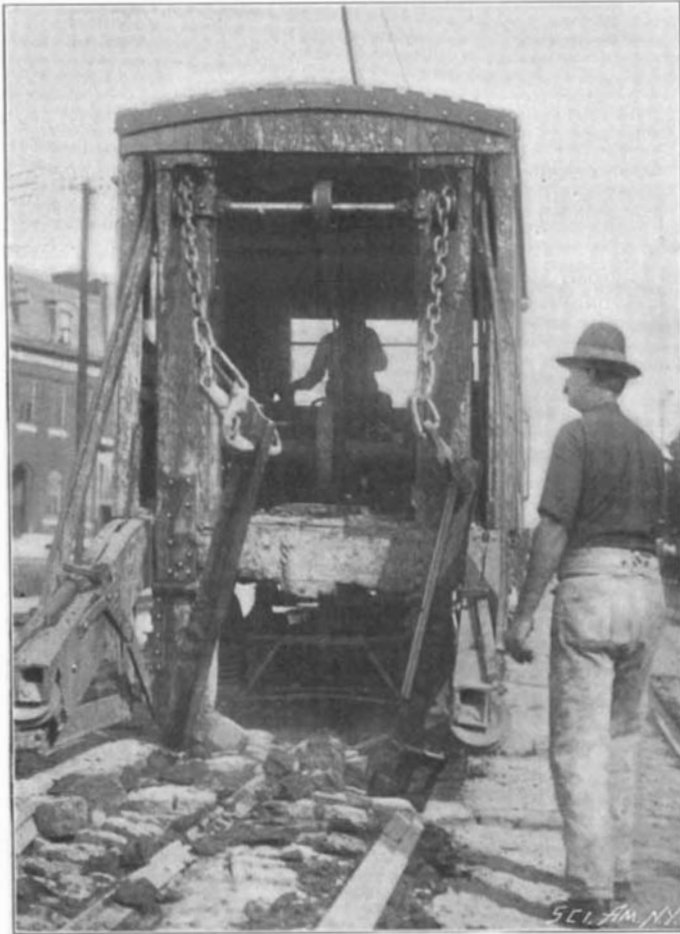
FRONT VIEW, SHOWING TWO LENGTHS OF RAIL PULLED LOOSE AND BROKEN.
