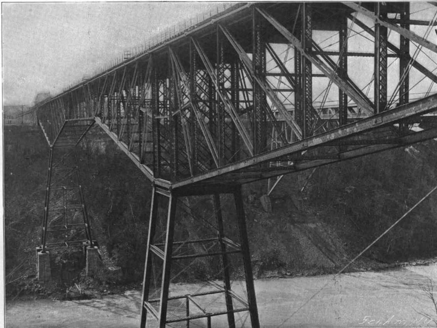
NIAGARA CANTILEVER BRIDGE BEFORE INSERTION OF NEW CENTER TRUSS AND TOWER COLUMNS.
