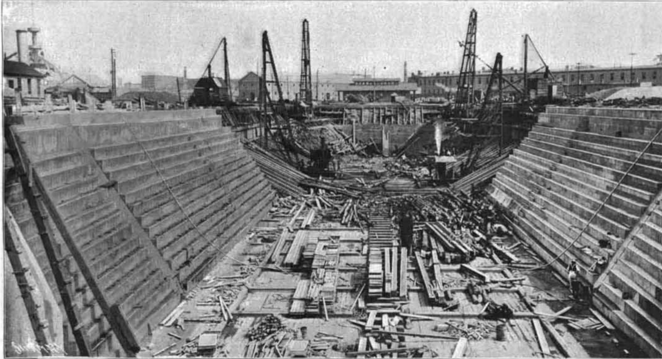
Width of floor of old dock, 50 feet; of new dock, 74 feet. View Showing One-half of Dock Reconstructed in Concrete.
