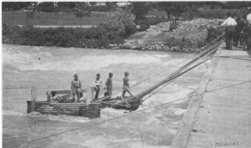
WORKMEN PREPARING A FOUNDATION FOR A NEW BRIDGE AT NIAGARA, WITHIN 500 FEET OF THE AMERICAN FALLS. LIFE-LINES ATTACHED TO THE WORKMEN.
