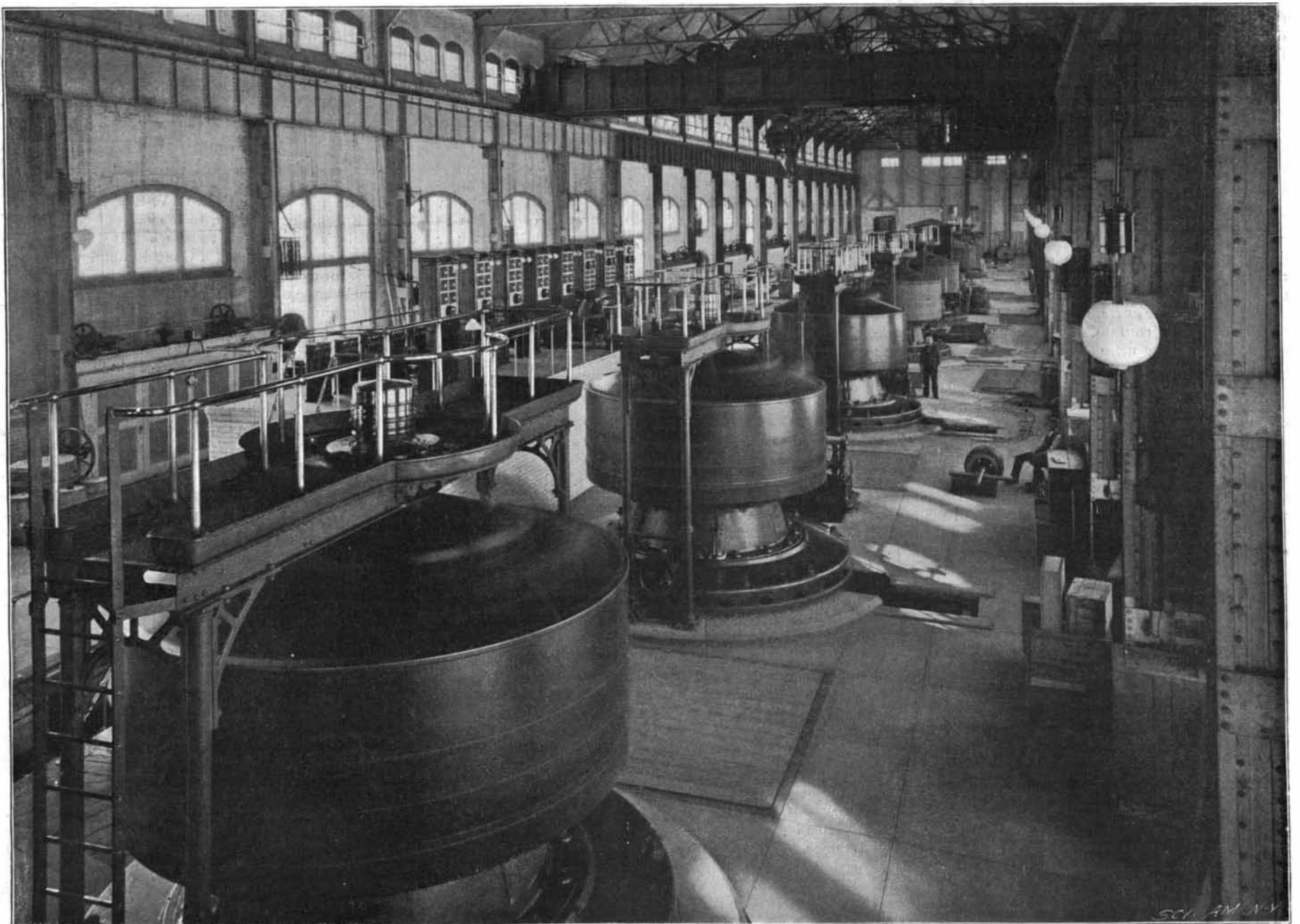
3.—The 50,000 H. P. Power House, with Eight 5,000 H. P. Generators Installed, NIAGARA FALLS POWER PLANT—III.—[See page 56.]
