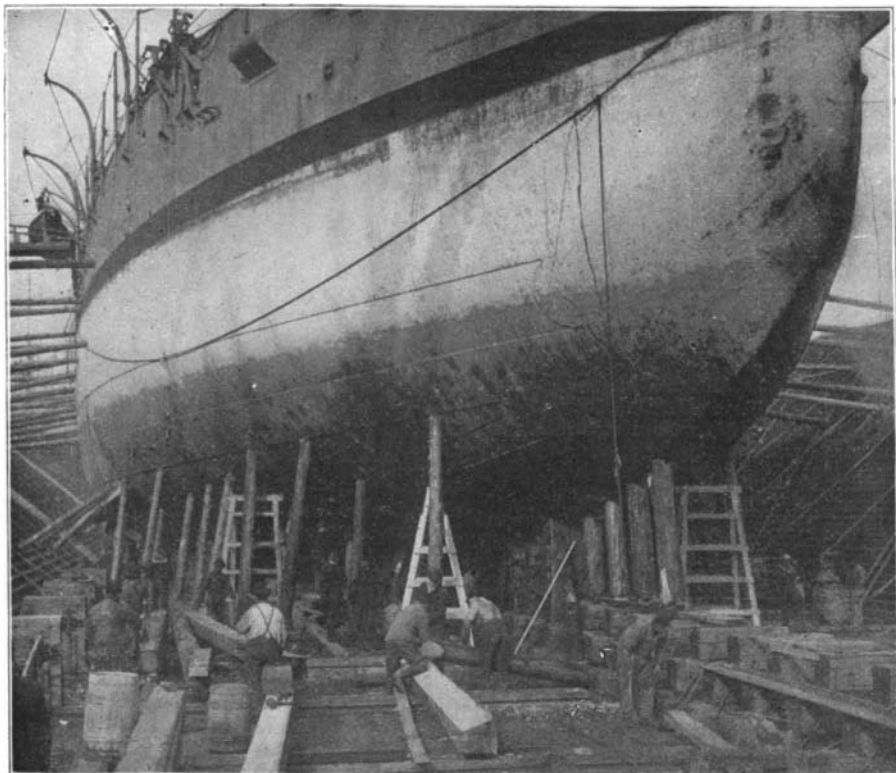
5.—Bow View of Ship when Water was First Pumped Out of Dock, Showing Method of Shoring.
