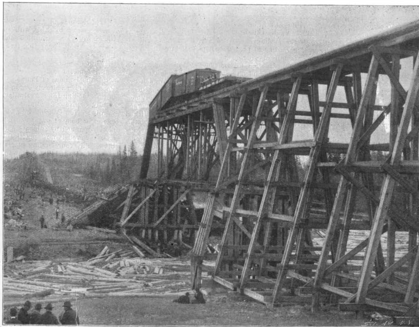
NEMADJI RIVER TRAIN WRECK—LOOKING FORWARD FROM REAR OF TRAIN.
